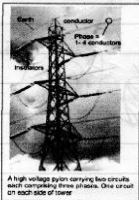
A high voltage pylon carrying two circuits each comprising three phases. One circuit on each side of tower
